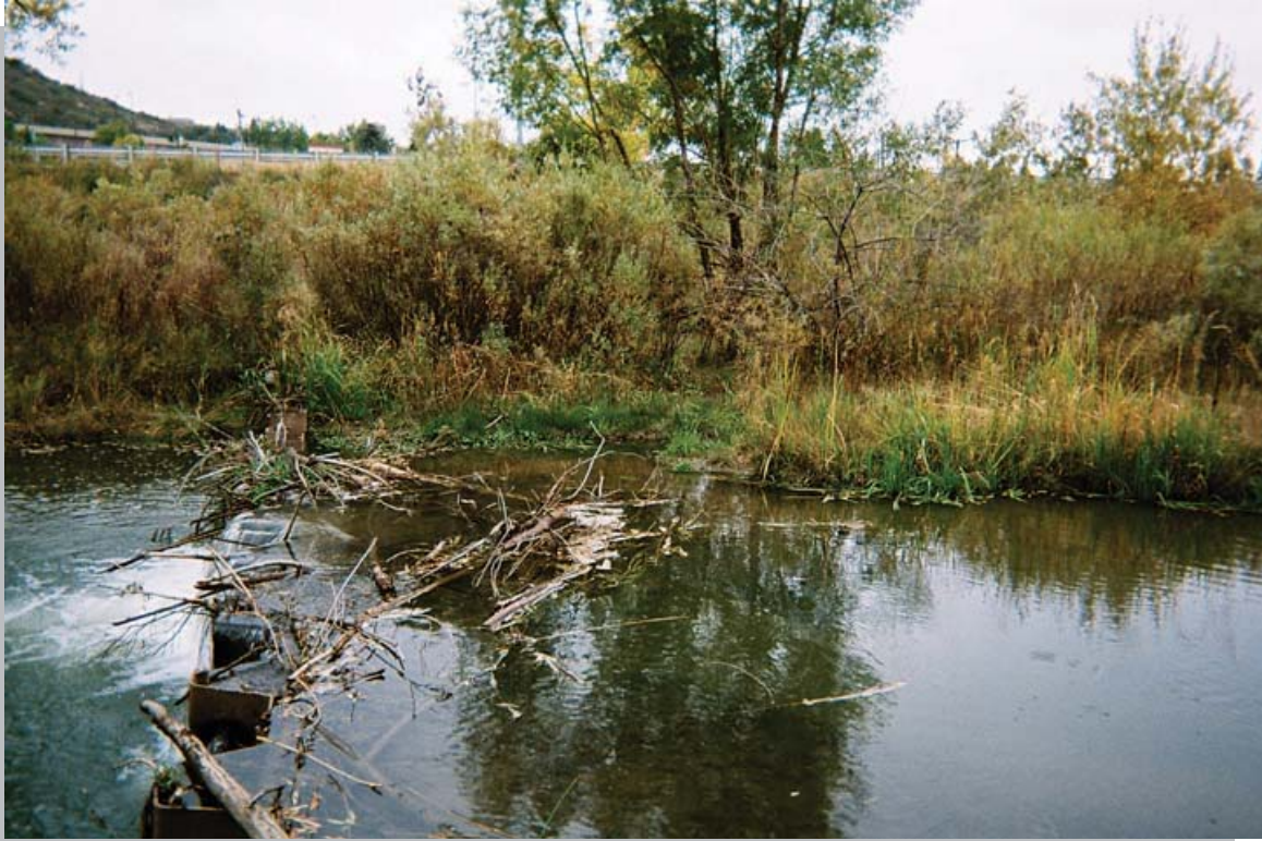
Figure 3 - Example of sheet pile cutoff drop structure on East Plum Creek in Castle Rock, Colorado used to enhance Preble's habitat.
