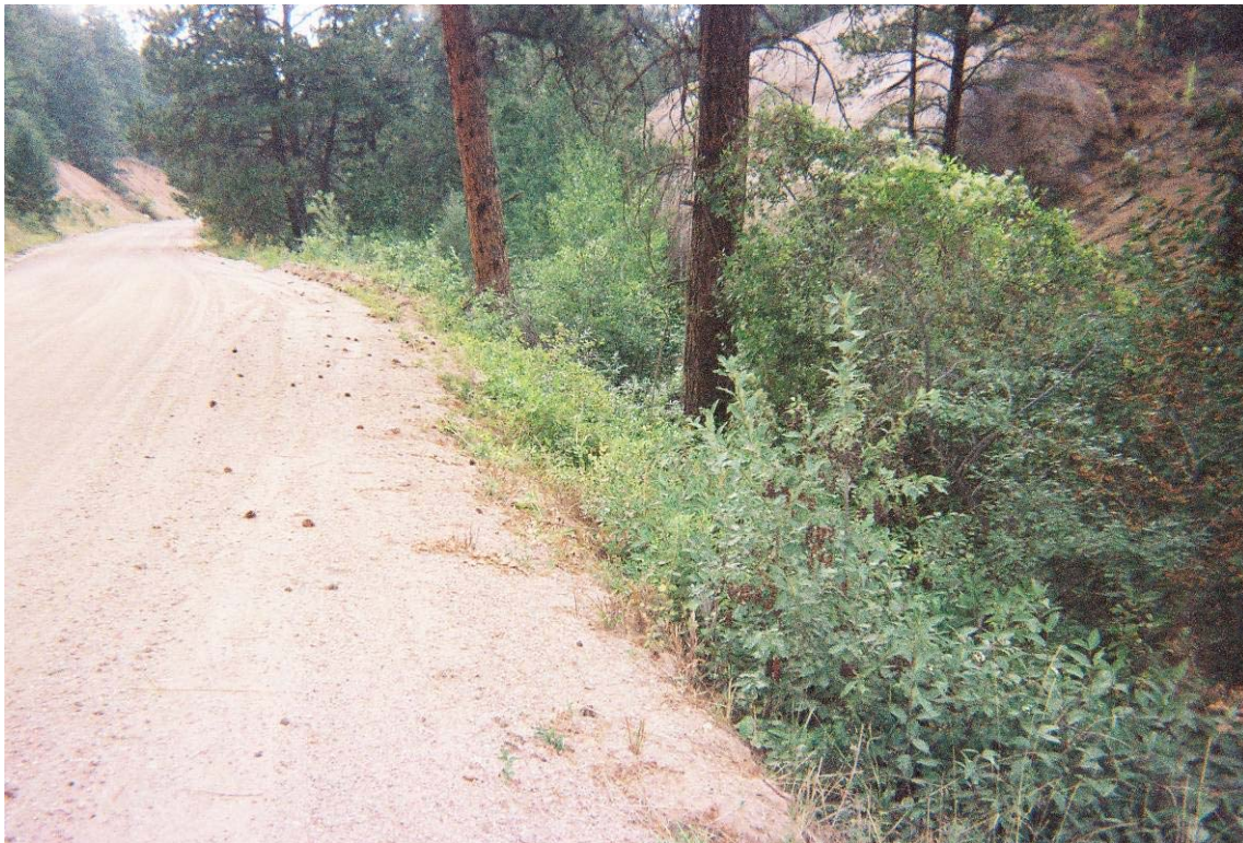
Photo H-5. Highway 67 eroding into Sugar Creek riparian zone.
