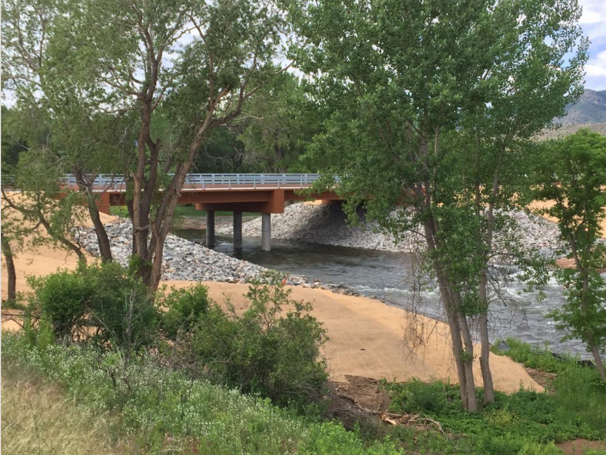
South Platte River Bridge following modifications to accommodate the new reservoir elevation of 5,444 feet.
