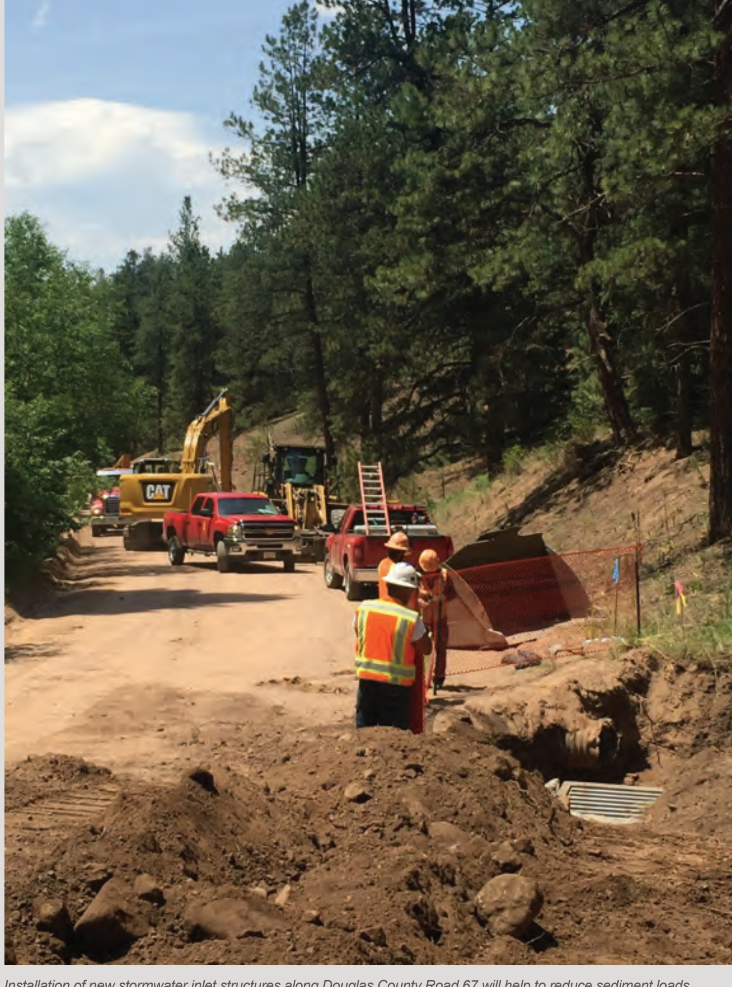
Installation of new stormwater inlet structures along Douglas County Road 67 will help to reduce sediment loads in the Sugar Creek drainage.
